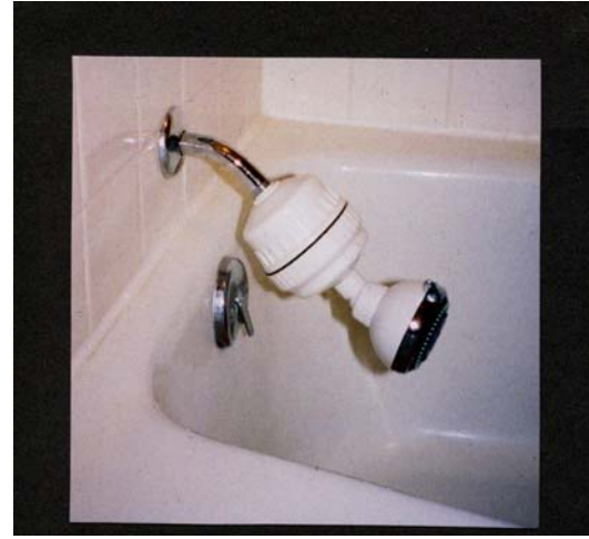
SIDE VIEW OF PIMAG SHOWER FILTER USED IN BATHTUB
